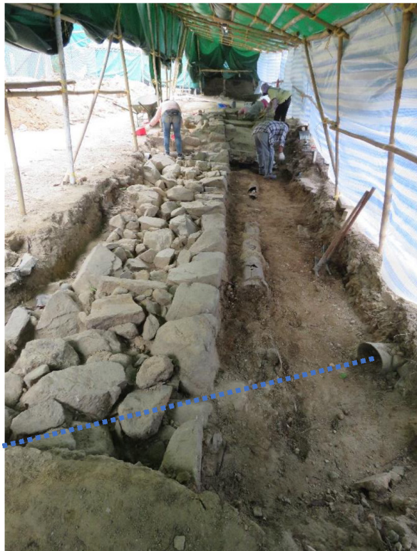
Figure 29 Excavation in progress showing ceramic pipe parallel to village wall and note partially removed plastic pipe [SF22] which extended over village wall; looking east.
