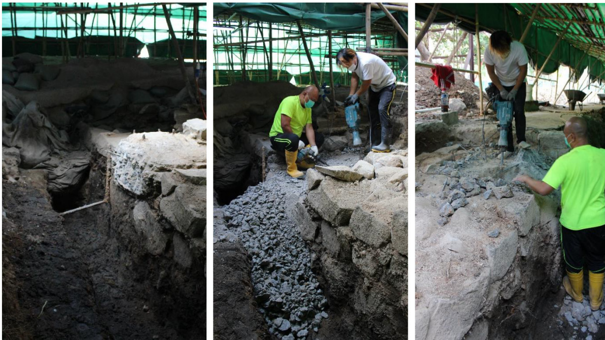
Figure 35 Concrete footing disturbing the village wall and removal of the concrete
