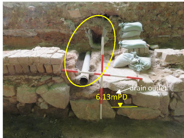
Figure 12 Modern drain and pipe are above and east of stone drain outlet at Lane 3; Looking south.
